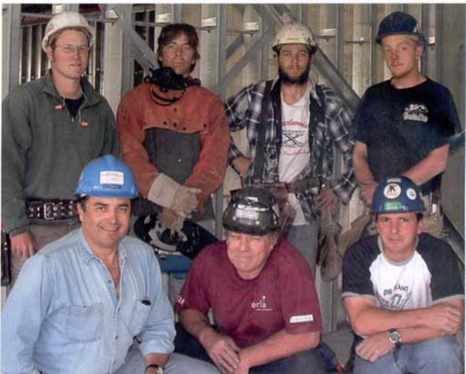
William Danshin (front left, in blue), with the Melit Steel Framing crew: Back row, L-R: Justin Crockett, Scott Hall, Shane Cameron, Jesse LeMasurier. Front row, L-R: Roy Fletcher and Kevin Turbide.
